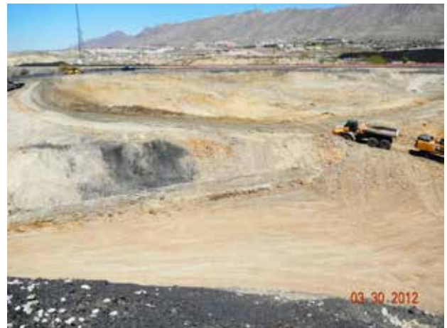
Loading of impacted soil beneath slag material within the PBA Interim Channel
