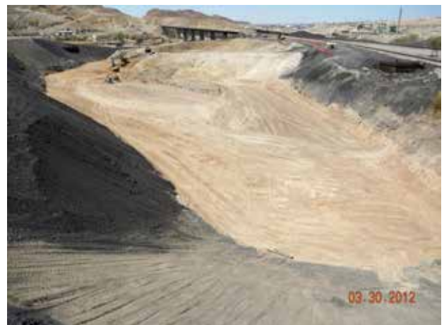
Excavation of impacted soil beneath slag material within the PBA Interim Channel
