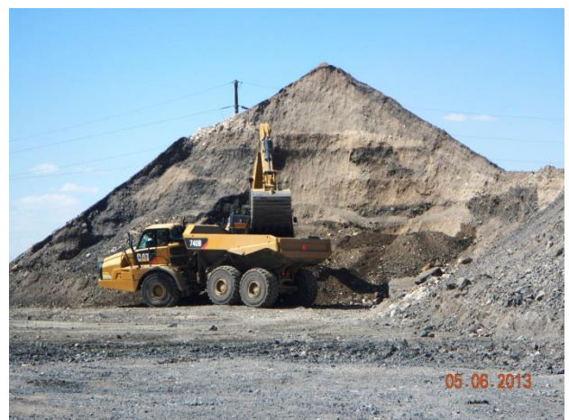
Loading CAT II materials to be relocated to the SW Fill Area
