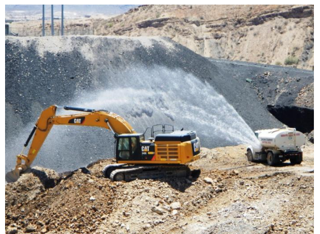
Excavation and loading of slag materials outside of the southwest corner of the Category 1 Landfill footprint.
