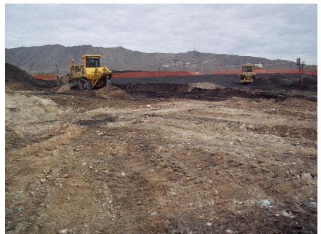
Ripping and stockpiling slag with a large bulldozer within Category 1 Landfill footprint.
