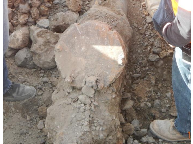
Existing sanitary sewer piping associated with future POTW Tie-In
