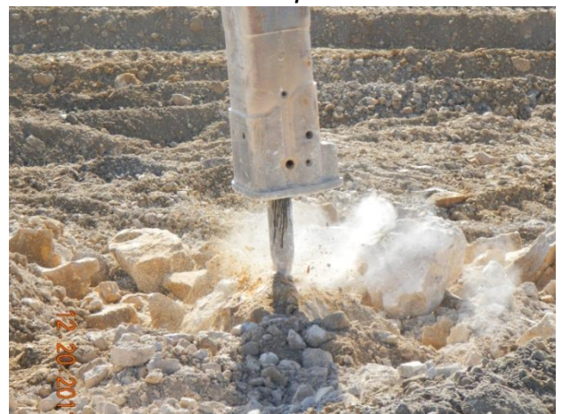
Breaking activities within the Category 1 Landfill footprint using a hydraulic breaker attachment and excavator.
