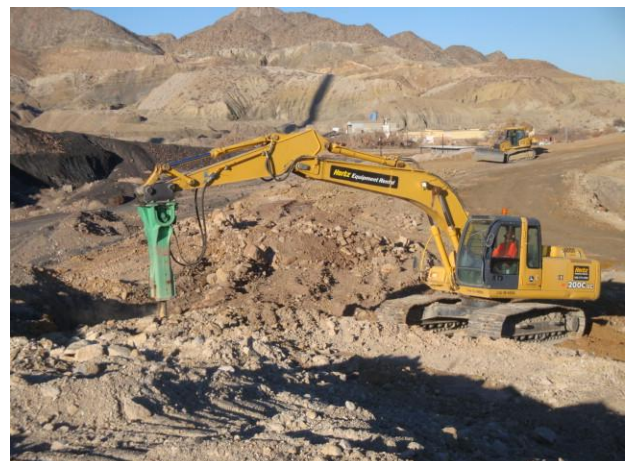
Breaking dense rock layer with a hydraulic breaker attached to an excavator.
