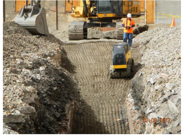
Compaction of the piping tunnel associated with the Engineering Trench using a remote controlled trench compactor
