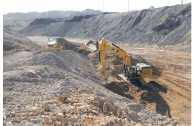
Excavation of impacted soil beneath slag material within the PBA Interim Channel
