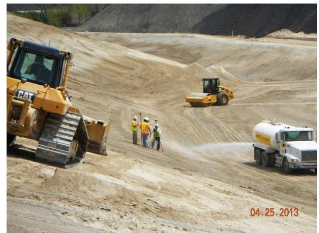
Moisture conditioning and grade confirmation of 6-inch prepared subgrade layer within Category 1 Landfill
