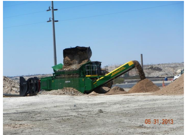
Screening of Category II material to produce protective layer material from Stockpile #2
