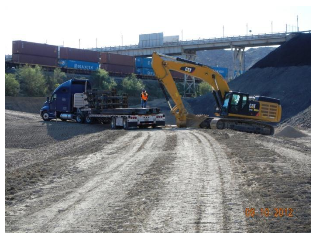
Offloading slide rail system near PRB 1
